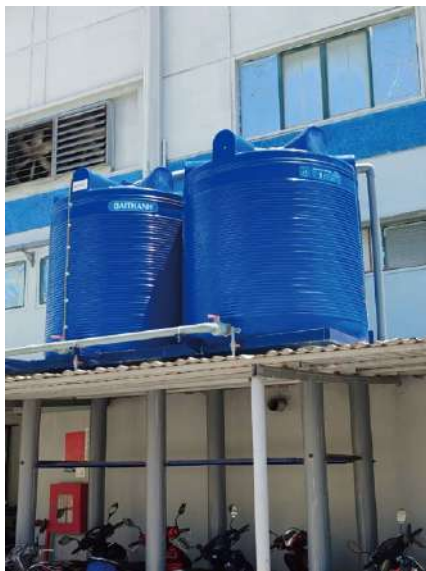
Recycle Water Storage Tank
